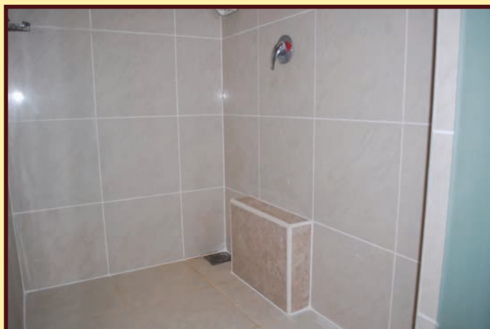
A new foot step in the shower cubicle in the male changing room at NSRCC Kranji
